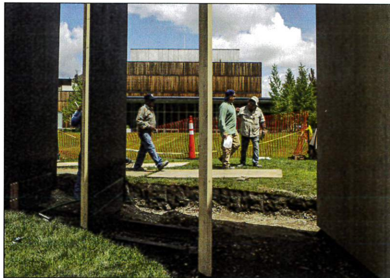
Work continues on the Town Enclosure last month on the Center for the Arts lawn. The grand opening starts at 5:30 p.m. tonight. The pavilion will have a longer lifespan than last summer's "Observatories" exhibition. The pavilion is available for free for nonprofits and artists to use at least through next summer.
